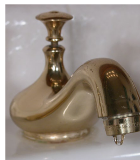
A chemical reaction causes solids to form in hot water pipes.
